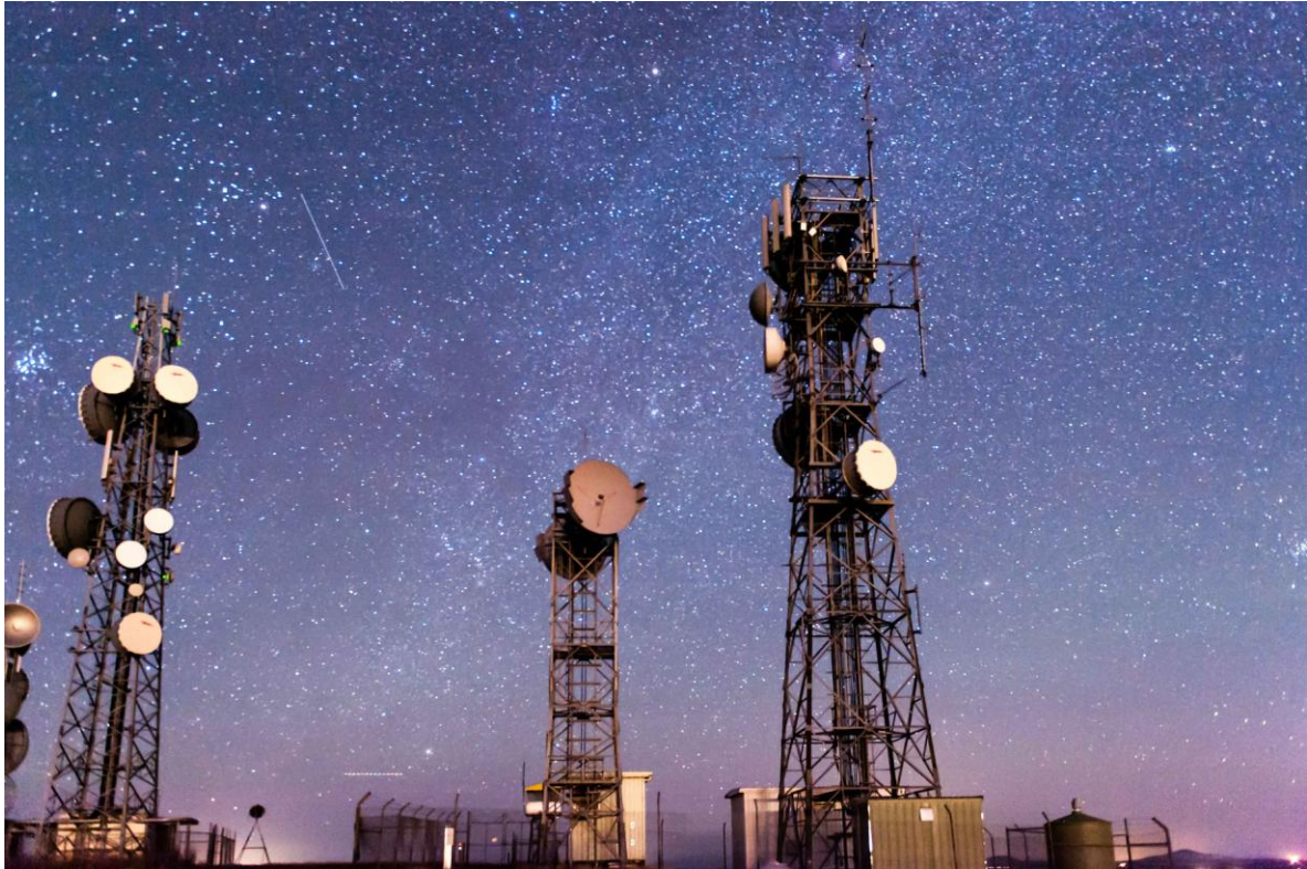
Communication Towers Mount Hollowback.
